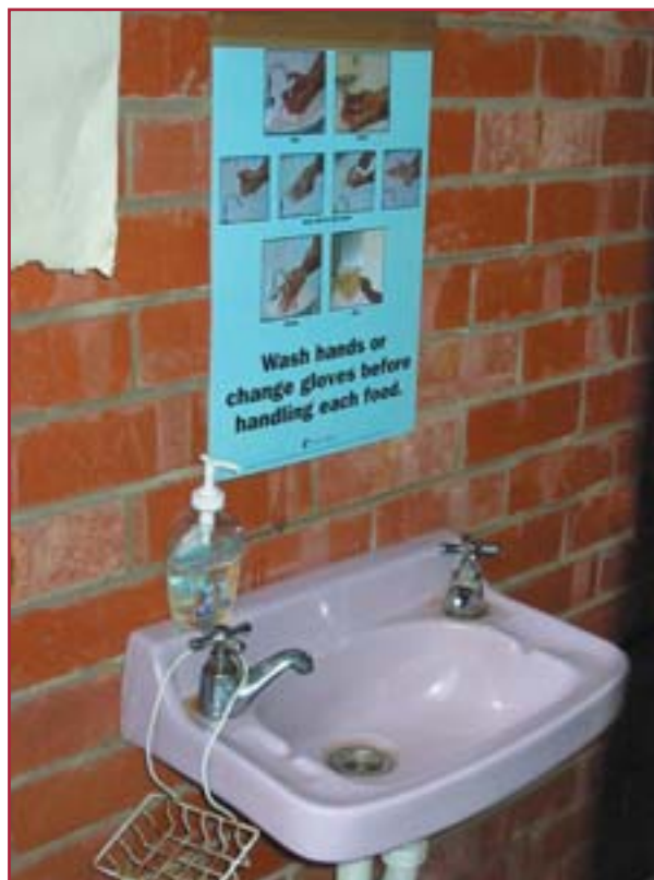
Photo 11. Hand washing facilities should be provided with instruction to employees
