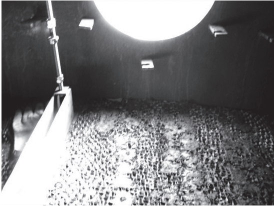
FIG. S1. Digital image showing the top portion of stainless steel matrix in the vacuum degasser unit through the manhole
